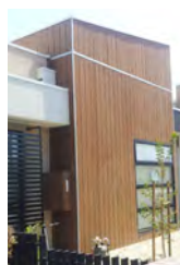
The board shows signs of lightening.
